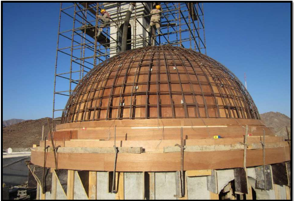
RAKJ-11 00 02 {Demolition & Re-Construction of Sheik Rashid Bin Saed Mosque at (RAK, AL FASHGA)}
