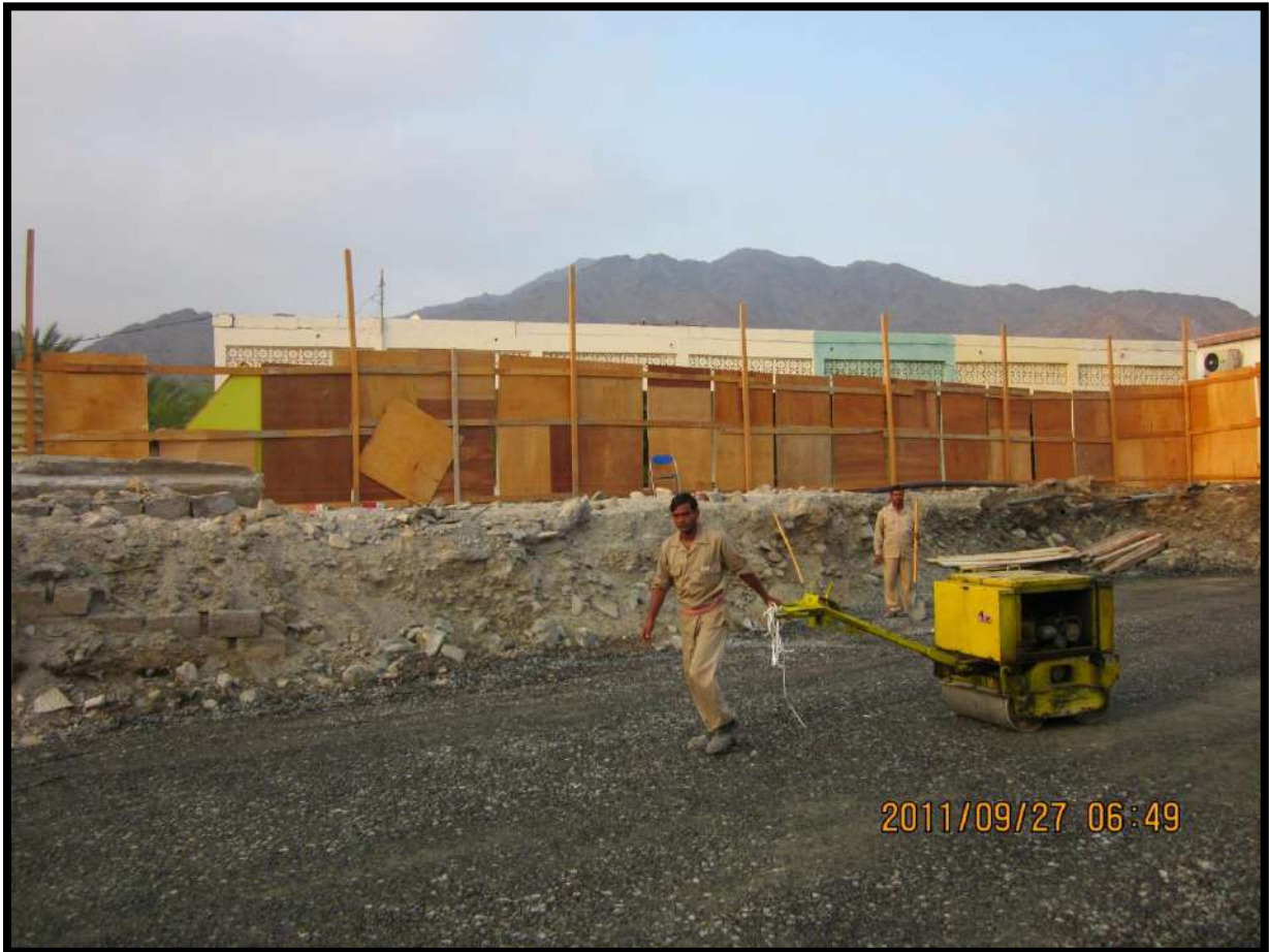
RAKJ-11 00 01 {Demolition & Re-Construction of Sheik Rashid Bin Saed Mosque at (RAK, AL Huwailath)}
